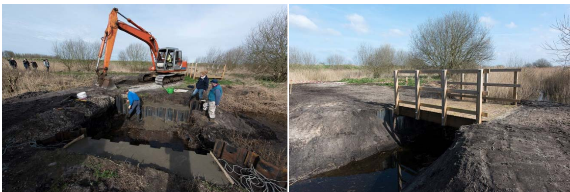
Image details by Dave Rogers: Infilling and levelling concrete for the bridge base (left), finished bridge with open channel running beneath, opening up access for fish connectivity between the two sites (right)
